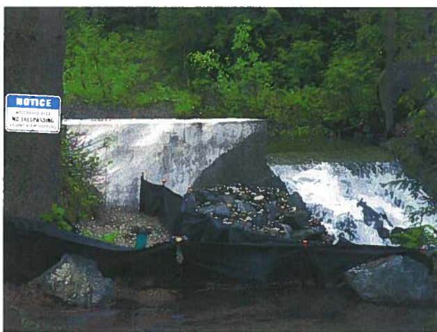
Topping Creek Raw Water Intake
